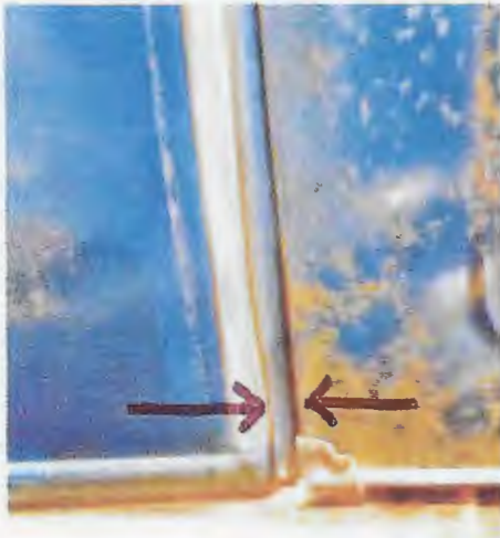
Above - This is where the hood does not fit properly; the gap is too wide due to a sagging bent frame.
